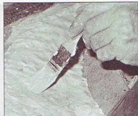
When the bottom coat of plaster has set overnight, the top finishing surface can be applied. Here it is being smoothed down with a dampened brush. The hexagons in the foreground are covered, but there are still plenty to be seen further along the embankment.
