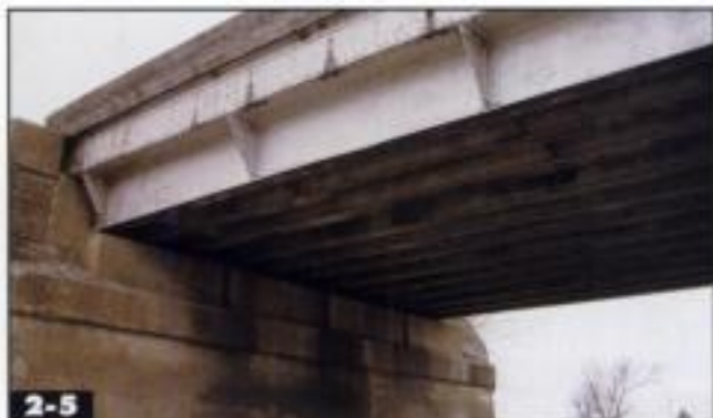
2-5 This double-track beam bridge has six steel I-beams under each track. Note the steel pieces that connect the I-beams, providing stability. Jeff Wilson
