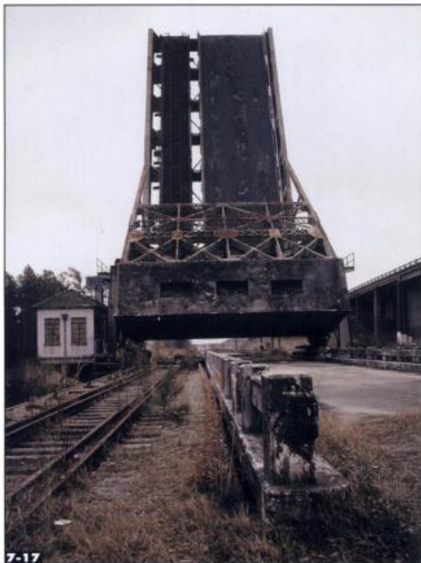
This out-of-service rolling lift bridge once carried highway traffic as well as Atlantic Coast Line trains over the Intercoastal Waterway into Myrtle Beach, South Carolina. Jeff Wilson
