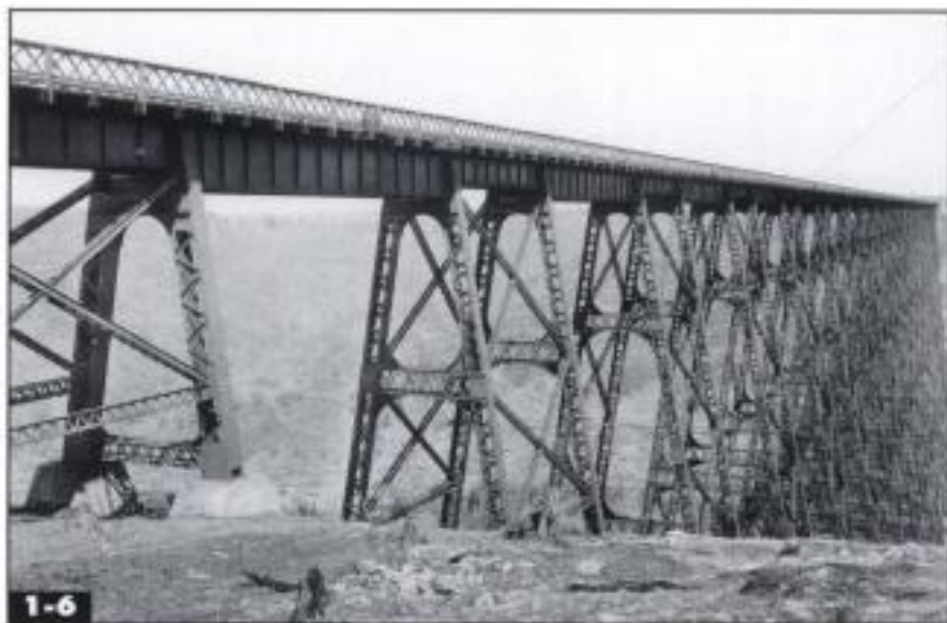
Since 1900, the steel viaduct has been the preferred way to cross wide valleys. Plate girder spans like this one are supported by steel piers. David P. Morgan Library collection
