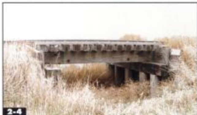
2-4 Used for short spans, wood beam bridges are basically trestles without bents. Jeff Wilson
