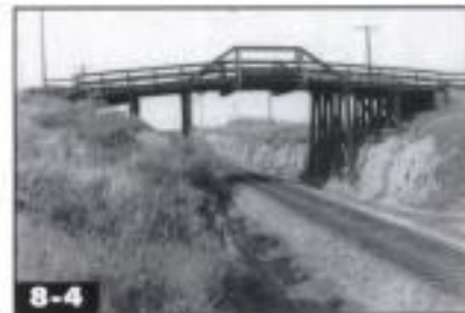
8-4 Queen-post bridges have a straight top chord with vertical hangers at each end. F.H. Bartholomew
