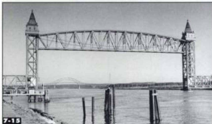
7-15 This 544'-long lift bridge carried the New Haven across the Cape Cod Canal at Buzzards Bay, Massachusetts. The bridge provides a 130' high clearance. With the bridge up, the counterweights are just above track level. Edward Ross
