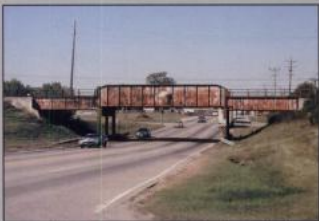
It's been a few years since this Chicago & North Western bridge has received a coat of paint. Jeff Wilson
