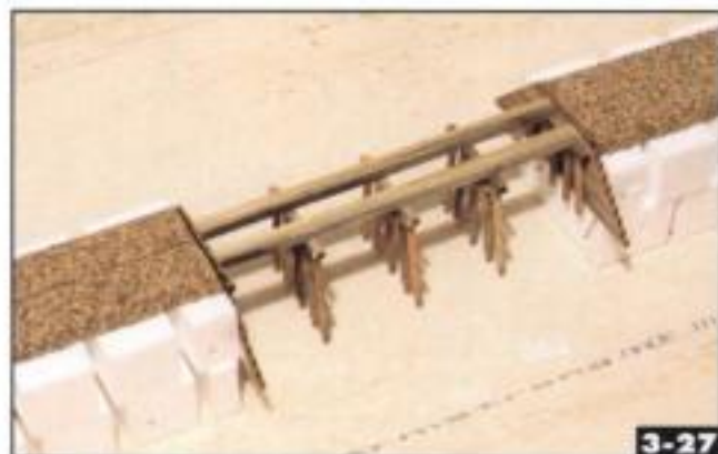
Test-fit the trestle. The top of the bulkhead wall should be less than a tie-thickness above the top of the roadbed. Jeff Wilson
