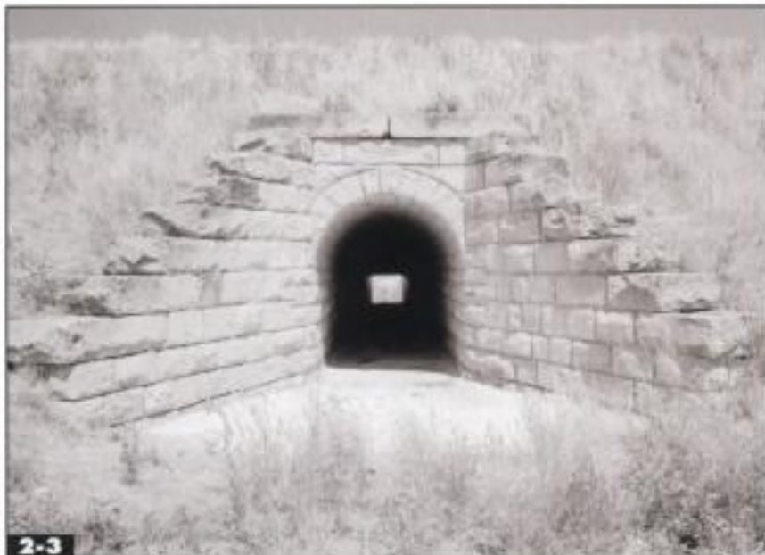
Stone culverts were built from the 1800s into the early 1900s. This culvert with wing walls is on the old Chicago & North Western line in Wyoming. Historic American Engineering Record; Jack Collier
