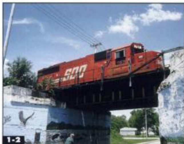
▲ This beam bridge is located on the former Soo Line at Sabula, Iowa. Extensions of the ties provide a base for the walkway. The concrete abutments make a handy canvas for a mural. Jeff Wilson
