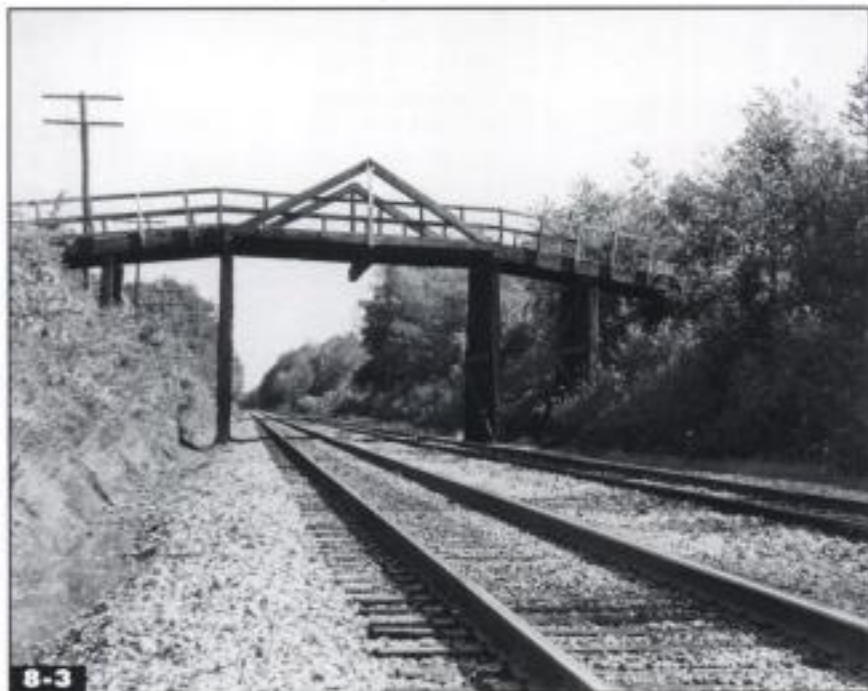
8-3 King-post bridges are simple trusses with a peak in the middle. Harold Russell
