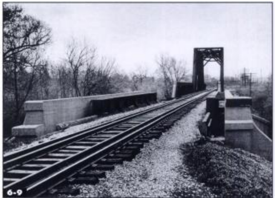
A view from above the Indianapolis Monon bridge reveals that the concrete girders are merely false fronts to a ballasted-deck plate girder span. Linn H. Westcott
