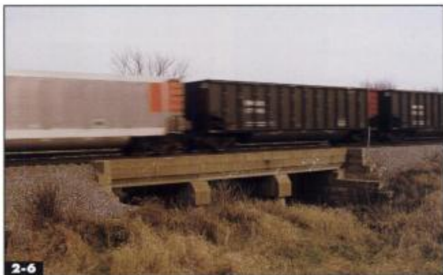
2-6 Concrete beam bridges are usually topped by a trough for a ballasted deck. This one is on the Union Pacific main line in Iowa. Jeff Wilson
