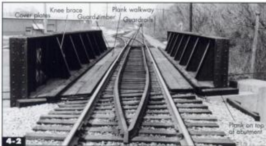
◀ Note how the ties on this skewed bridge are angled where the bridge meets the abutment. Sy Dykhouse
