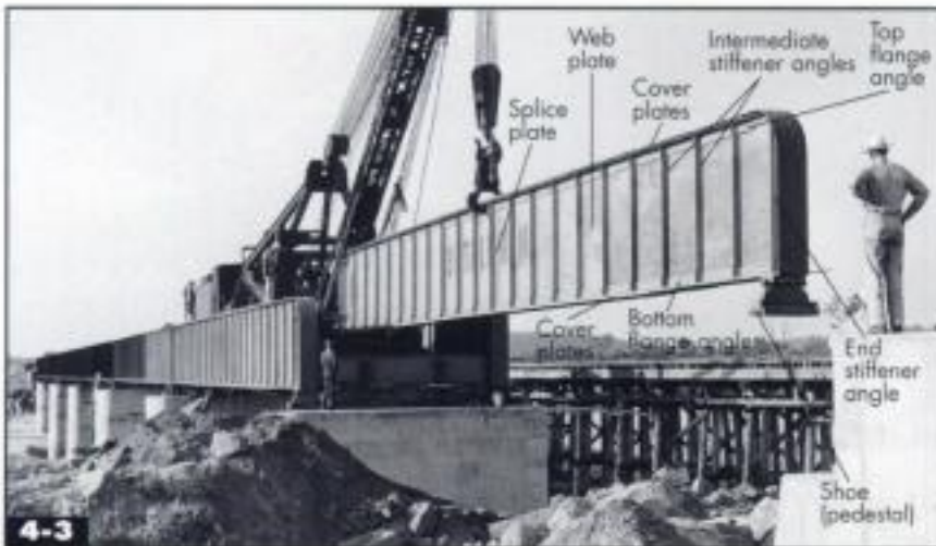
The components of this plate girder are in plain view as it is lowered into place. Missouri-Kansas-Texas Railroad
