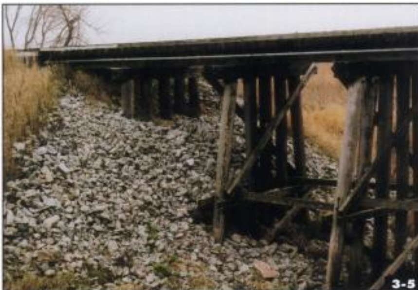
The posts on a pile trestle are driven directly into the ground, and therefore don't require footings like frame trestles. Jeff Wilson
