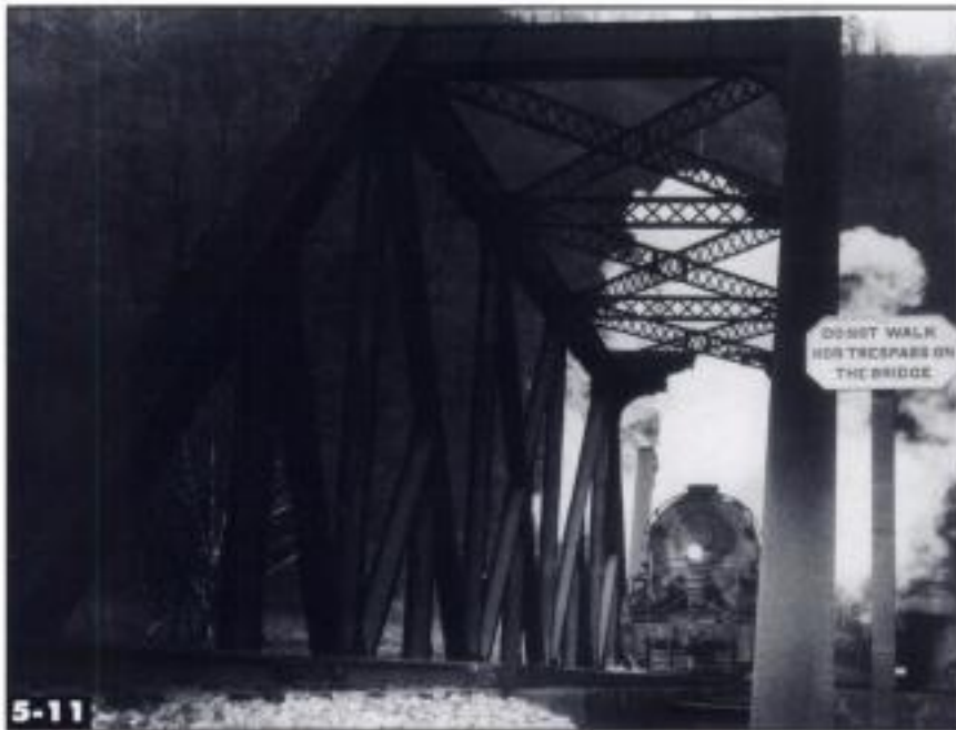
Baltimore trusses are a version of the Pratt (note the diagonals) with subdivisions. Rusty Ball
