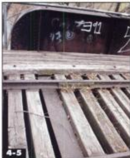
Note how the wood ties straddle the steel floor beam, which is taller than the stringers that the ties rest upon. This through-girder bridge has rounded corners. Jeff Wilson
