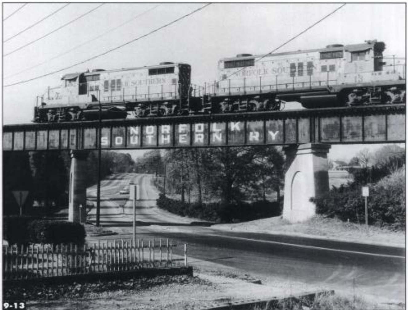
9-13 The eye-catching arch-pattern concrete piers under this skewed Norfolk Southern plate girder bridge would make distinctive scratchbuilt models. Curt Tillotson, Jr.
