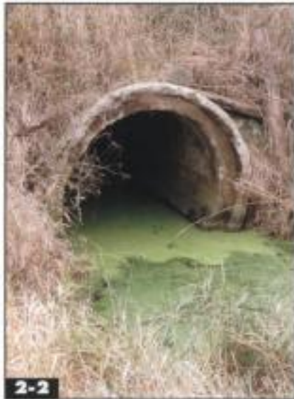
This concrete pipe is typical of the simplest culverts along railroad rights-of-way. Culverts are also made from corrugated metal, iron, and clay pipes. Jeff Wilson
